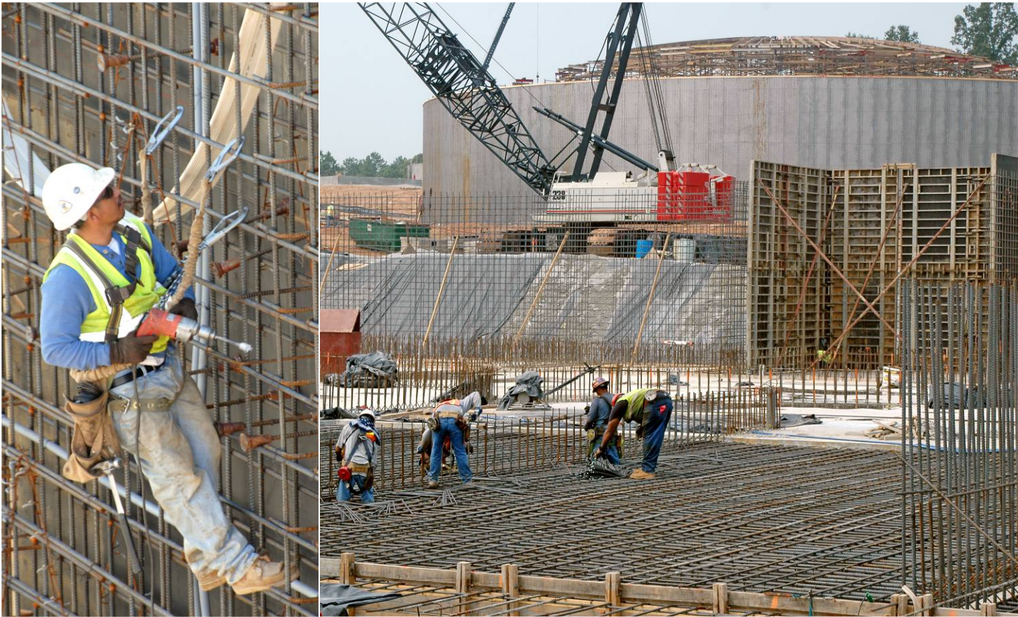
South Central Wastewater Treatment Plant – a USD 52 million project in Douglas County, GA.
